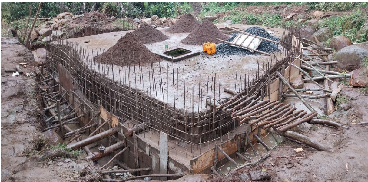
Renovation of spring capturing: initially made by government but almost became out of use
