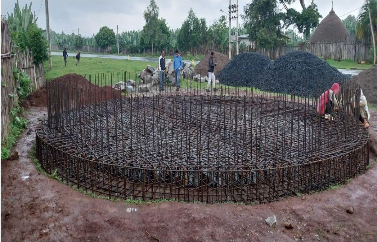
The beginning phase of water tank (reservoir): the volume of the tanker is 250 m 3 constructed along the road side.
